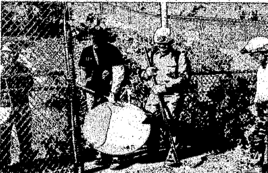
CAVERS SHOW THE TOOLS they will use to mix cement to install the newest gate inside Fort Stanton Cave Saturday, Oct. 23. The covers are shown at the above-ground gate and fence that surrounds the sink-hole that is the cave's entrance. Cavers from 8 New Mexico and Texas "grotsos" and members of the Lincoln County White Mountain Search and Rescue participated in the gate installation.
