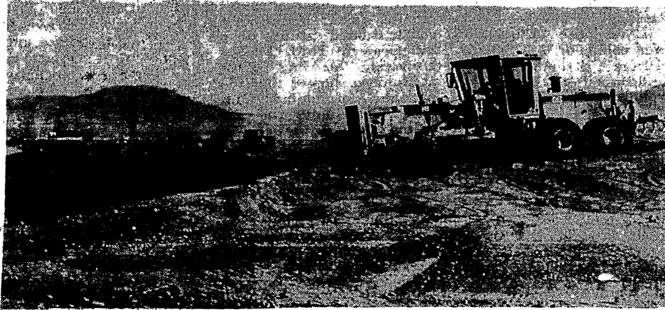
FINISHING TOUCHES. A Mountain States Constructors Inc. motorgrader finishes the shoulders on the new stretch of Highway 54, north from the intersection with Highway 380 in Carrizozo. The construction company raised and widened about three miles of the highway, which is a major north-south route in central New Mexico.
